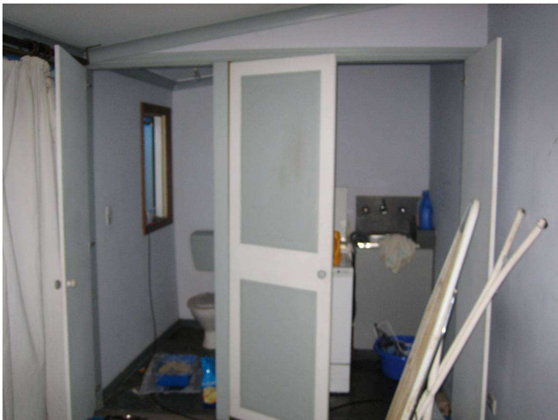
Toilet and Laundry facility in sleep-out area.
