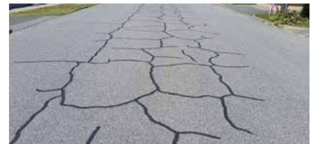
AN INTERIM CRACK SEALING, OR PREVENTATIVE MAINTENANCE, TO EXTEND THE LIFE OF THE ASSET (FLEET ST – ACCESS ROAD)
