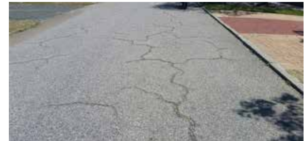
AN EXAMPLE OF LONGITUDINAL REFLECTIVE CRACKING (CORONATION STREET – ACCESS RD)
