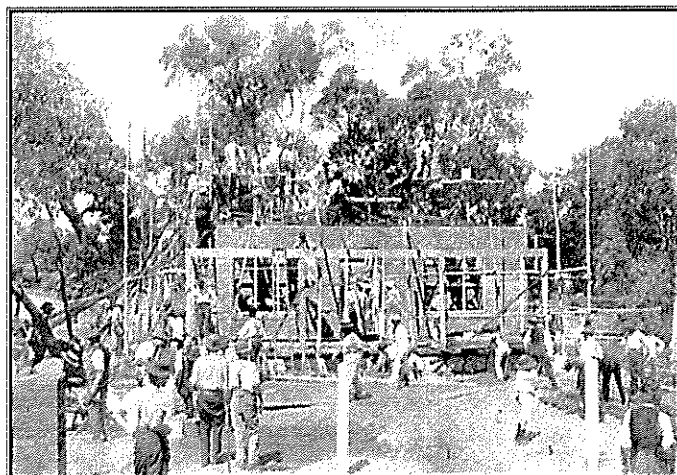
Building Anzac Cottage- Progress made by the "Busy Bees" up to 2 pm
