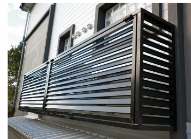
WALL MOUNTED UPPER FLOOR AIR-CONDITIONING SCREEN
