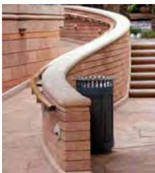
Universal access facilities is to be attractive and well integrated into the design of any development.
