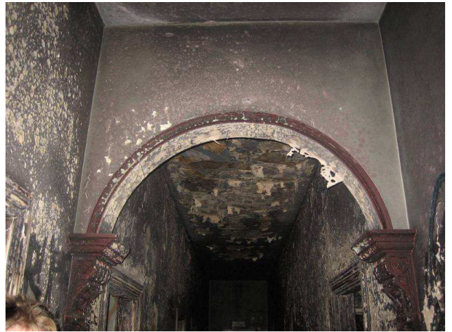
First Floor Corridor Archway - Evidence of Fire Damage
