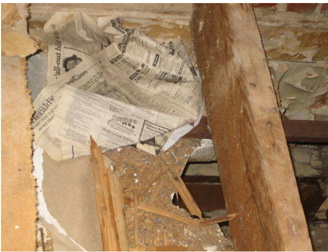
Evidence of White Ant Activity - First Floor
