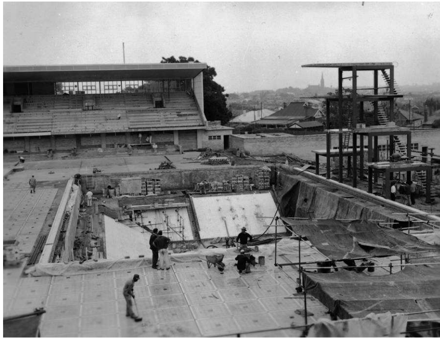
Photo 5 City of Perth Aquatic Centre, Beatty Park, under construction, Batty Library Pictorial Collection BA 1103-29. n.d.
