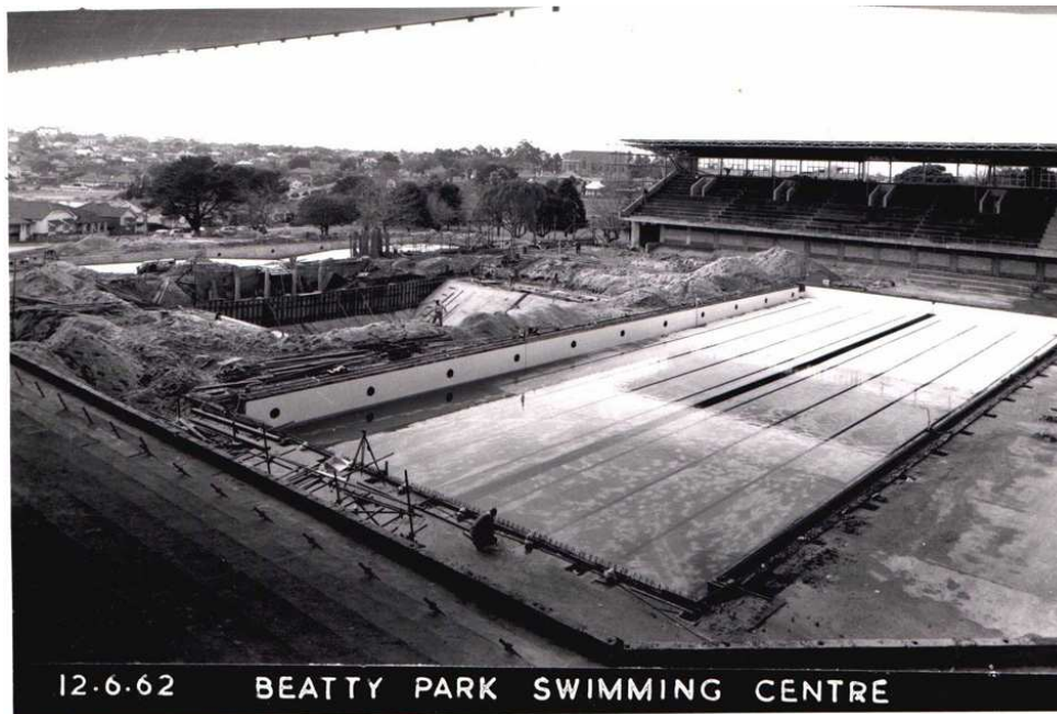
Photo 6 Aquatic Centre, Beatty Park , 12 June 1962, courtesy Town of Vincent Library. Note work to date on spectator stands, main pool and diving pool.
