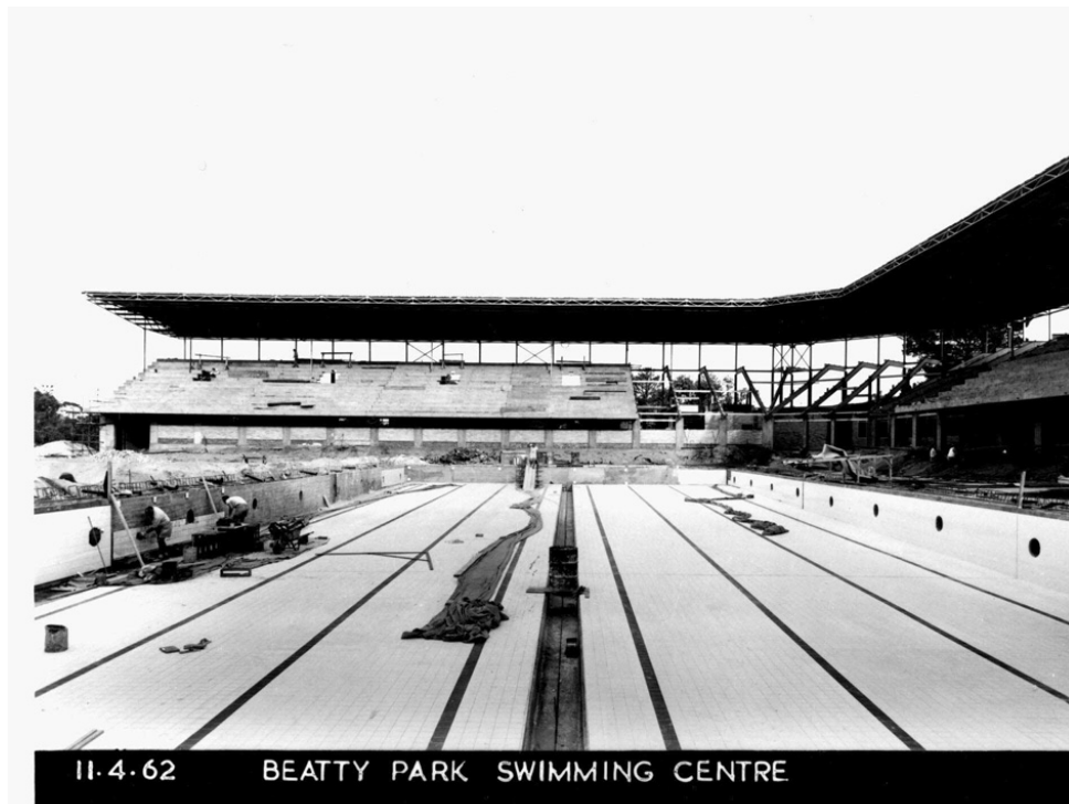
Photo 3 Aquatic Centre, Beatty Park , 11 April 1962, courtesy Town of Vincent Library, showing construction of pools and spectator stand.
