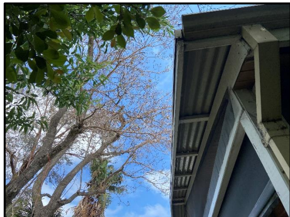
Image taken by Arbor Centre facing West – showing failed stem caught in canopy
