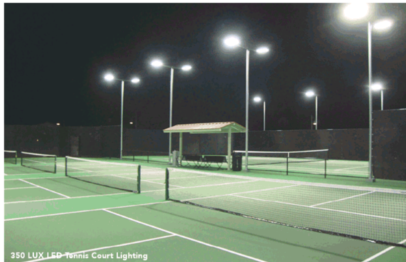
350 LUX LED Tennis Court Lighting
