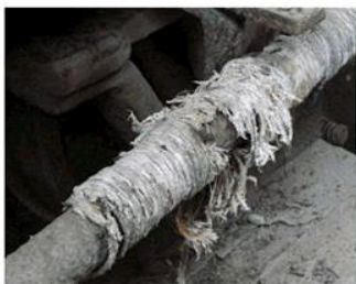
Broken ACM pipe
