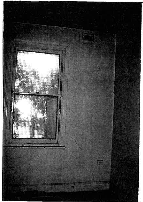
Photograph 29 Lee Hop's Cottage Rear bedroom (south west) wall cracks.
