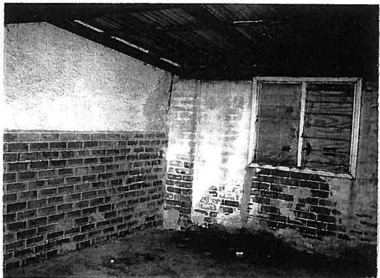
Photograph 20 Lee Hop's Cottage Garage interior showing cottage wall and deterioration of the garage wall.
