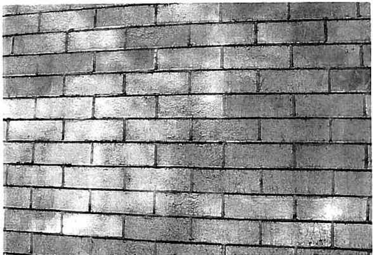
Photograph 47 Halvorsen Hall Wall detail (northwest) showing brick damage
