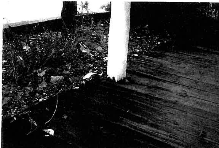
Photograph 23 Lee Hop's Cottage Front verandah subsidence.
