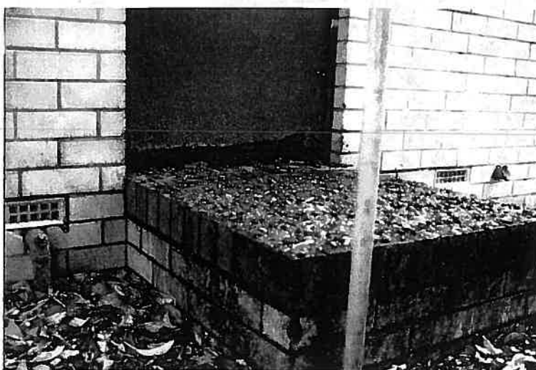
Photograph 49 Halvorsen Hall South west entry-dangerous condition.
