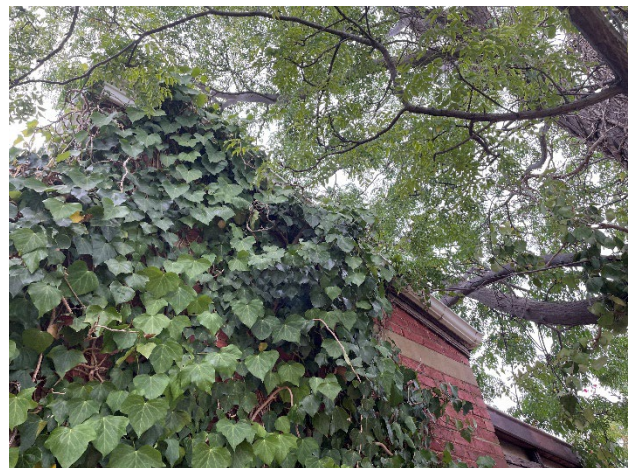
Figure 33: Overgrown creeper on the west elevation.
