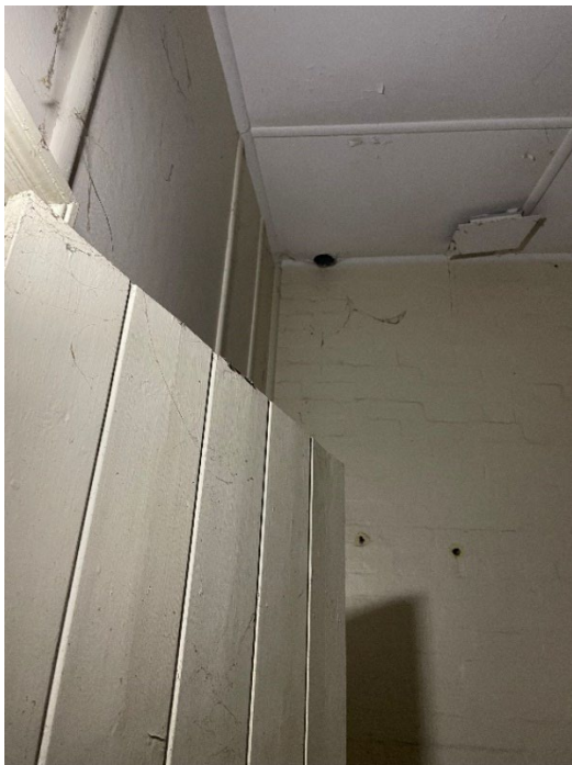
Figure 62: Bathroom door and ceiling.
