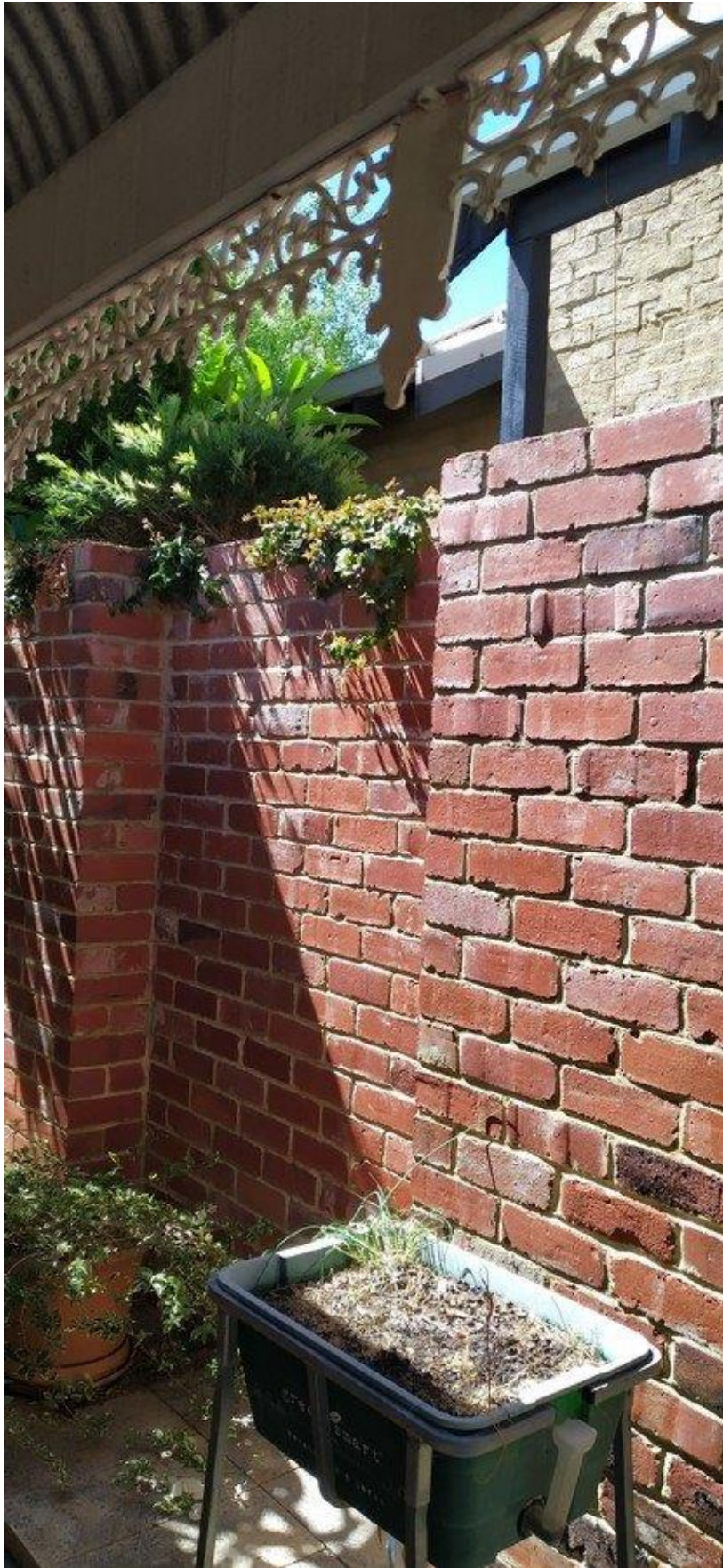
Figure 5: Existing bullnose verandah and boundary fence of 57 Glendower St providing visual cut-off and limiting field of view to adjoining property at 4 Primrose St
