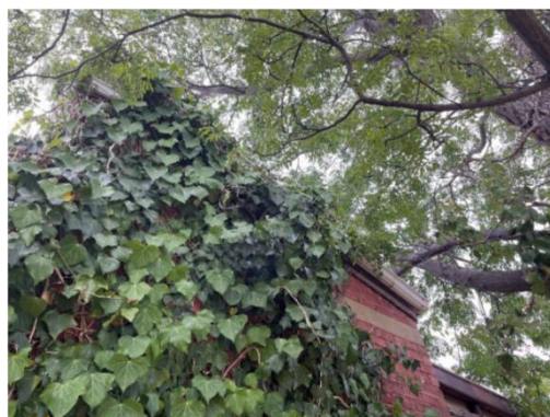
Figure 33: Overgrown creeper on the west elevation.
