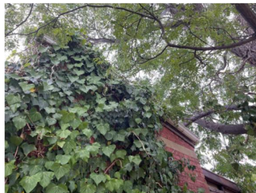
Figure 33: Overgrown creeper on the west elevation.
