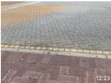
Painted colours on road are extremely faded and not very noticeable
