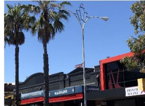
Art Deco Street Lights between Chelmsford Road and Walcott Street do not provide adequate light and will be upgraded in 2022/23.
