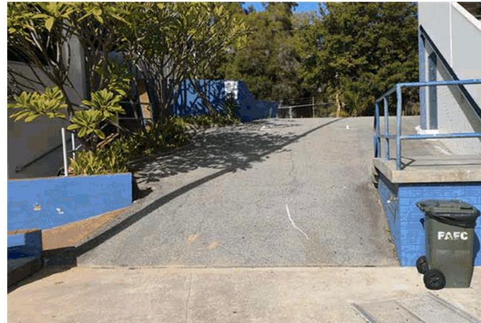
Access grades non-compliant
