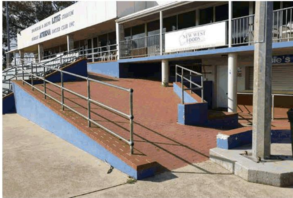
Access grades non-compliant
