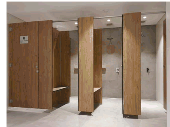
Indicative Shower Cubicle Design Plumbing Fixtures as per City of Vincents' Standard Specification
