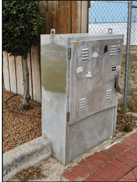
Figure 3 – Electrical Service Box
